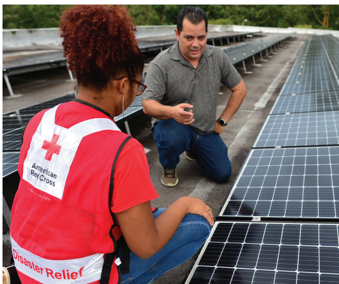
At the Angelita Delgado Sella School in Lares, teacher Ramón Arroyo and a Red Cross worker discuss the positive impact of a newly installed solar micro-grid system. Photo by the American Red Cross.
